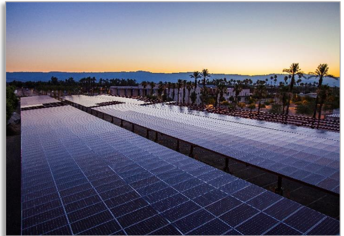
Solar Photovoltaic System
