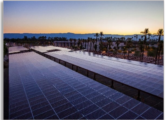
Solar Photovoltaic System
